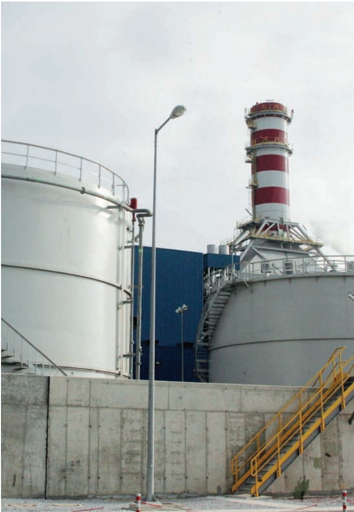
Unit of electricity production with natural gas (in Thessaloniki)
